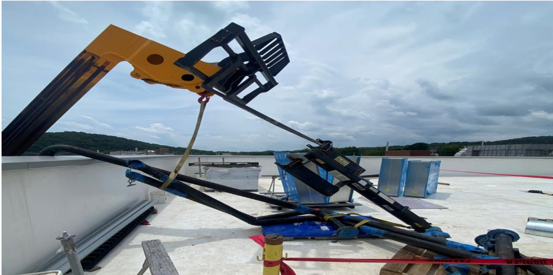
Telehandler, Jib, and Load on Roof Post-Incident
