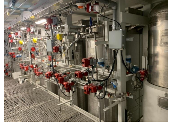
Tank Side Cesium Removal System Process Enclosure
